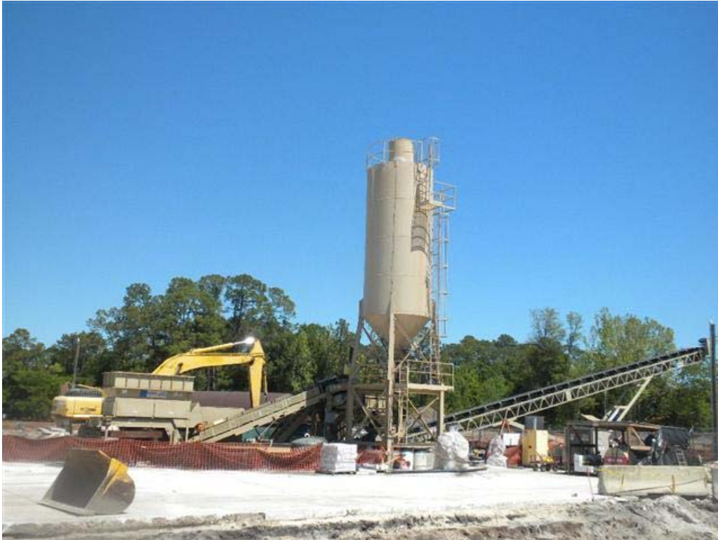
Pugmill, Silo and Conveyor
